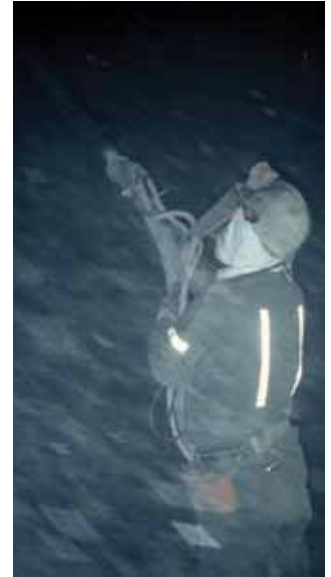
Poorly illuminated, dusty and dirty conditions are not conducive to a safe, efficient, high quality shotcrete operation.
