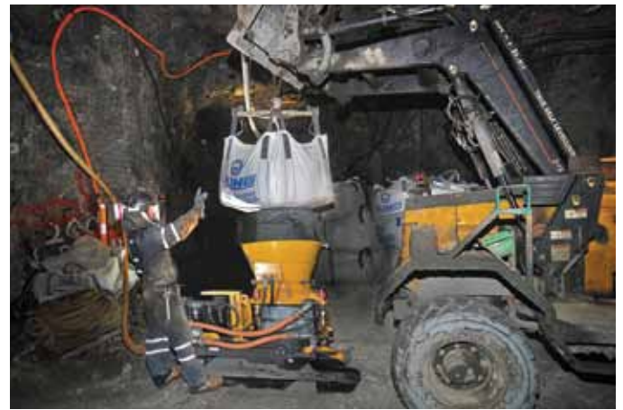
Hopper hoods serve the dual purpose to protect the operator's hands in the event of a bag drop and also to prevent excess amounts of nuisance dust from escaping into the atmosphere.
