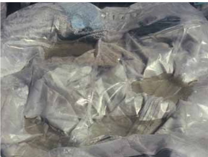
If shotcrete bags are left unprotected, rainwater will accumulate and can easily permeate through the polycover, and hydrate chunks of shotcrete.
