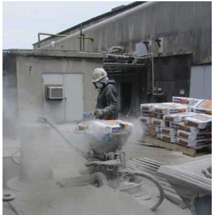
In a dry-mix shotcrete application, a major point of dust generation is the delivery hopper (also applies to the use of pre-packaged materials in a wet-mix operation).
